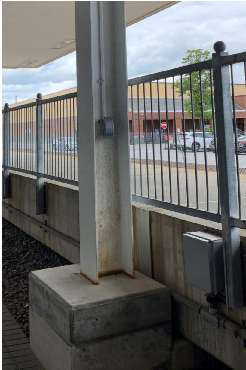
COLUMN BASE PAINT FAILURE AND CORROSION
