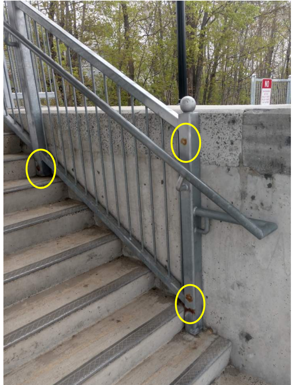
ISOLATED COATING FAILURE ON METAL RAILING
