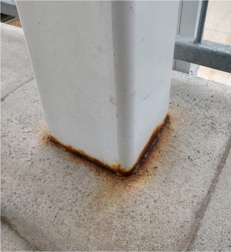
COLUMN BASE PAINT FAILURE AND CORROSION
