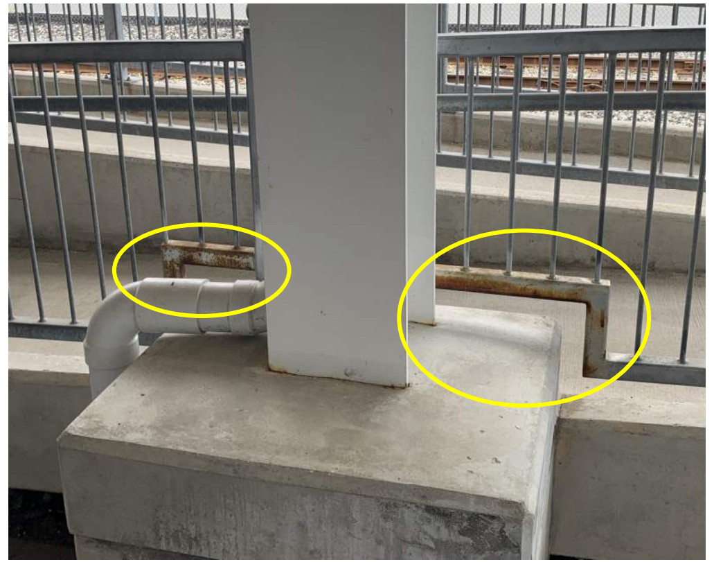
ISOLATED COATING FAILURE ON METAL RAILING
