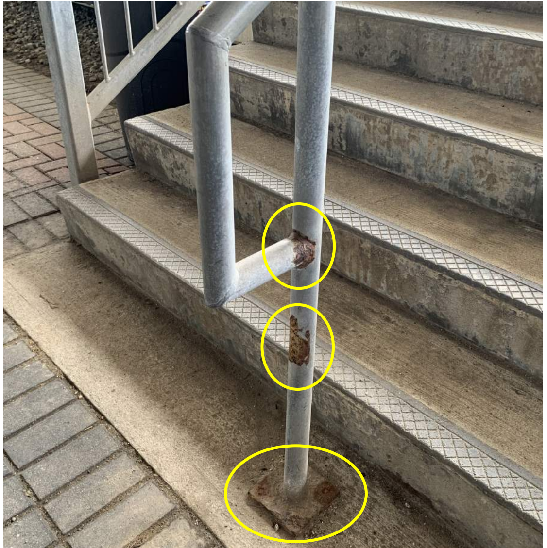
ISOLATED COATING FAILURE ON METAL RAILING
