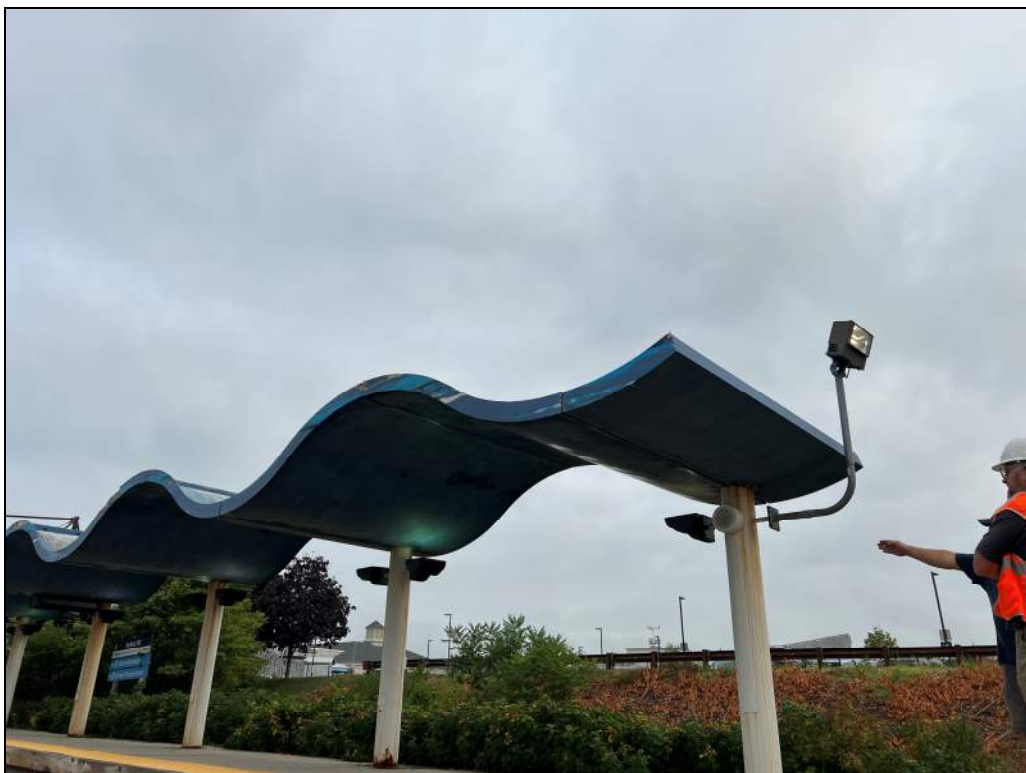
Photo 2 – Light Fixture at End of Canopy (to Remain)
