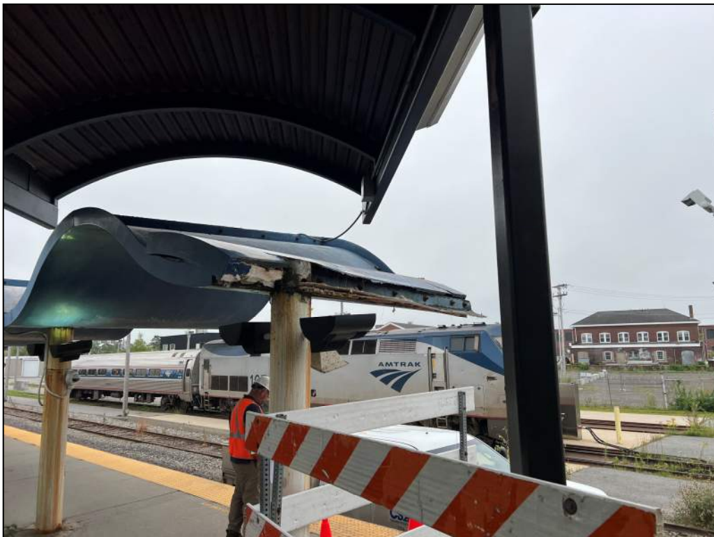
Photo 4 – Damage to Existing Canopy Adjacent to Trainway
